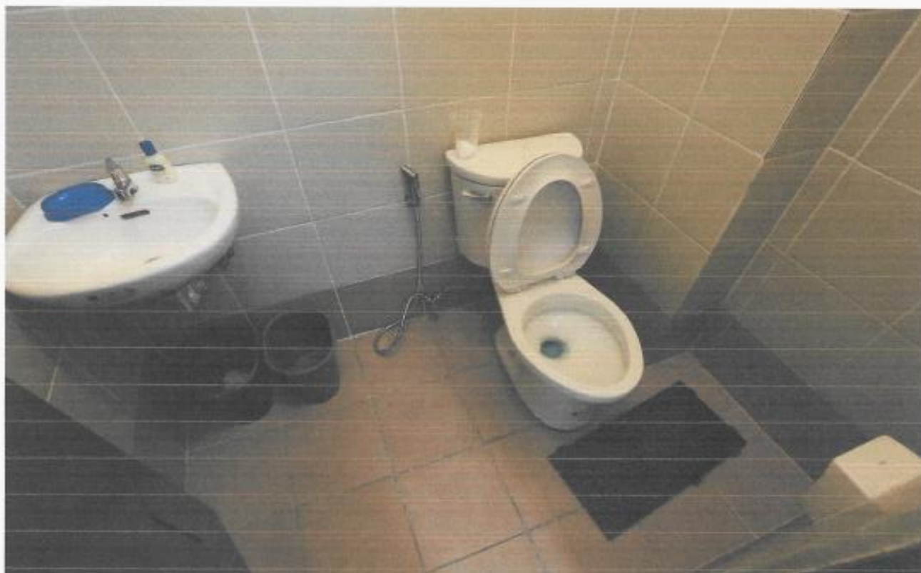
CEA MEDICAL TOILET
